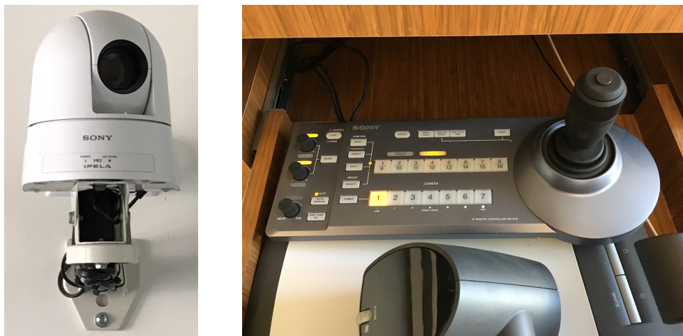
Figure 2. The camera is attached to the rear wall of the classroom and controlled by a joystick/keypad device located in a cabinet located inside a podium at the front of the classroom.
