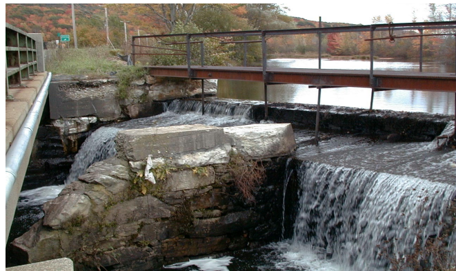
Figure 6. The dam on the north end of the North Basin of Hoosac Lake in its current state of disrepair.
